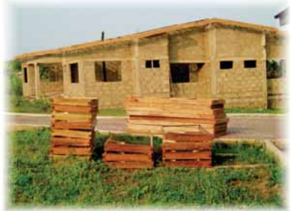
New Life Baptist Church: Bible Institute and Guest House building under construction in Mumford C/R.
